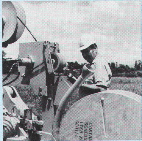
Checking the optical-fibre cable as it passes through the laying tube into the ground near Perth.
